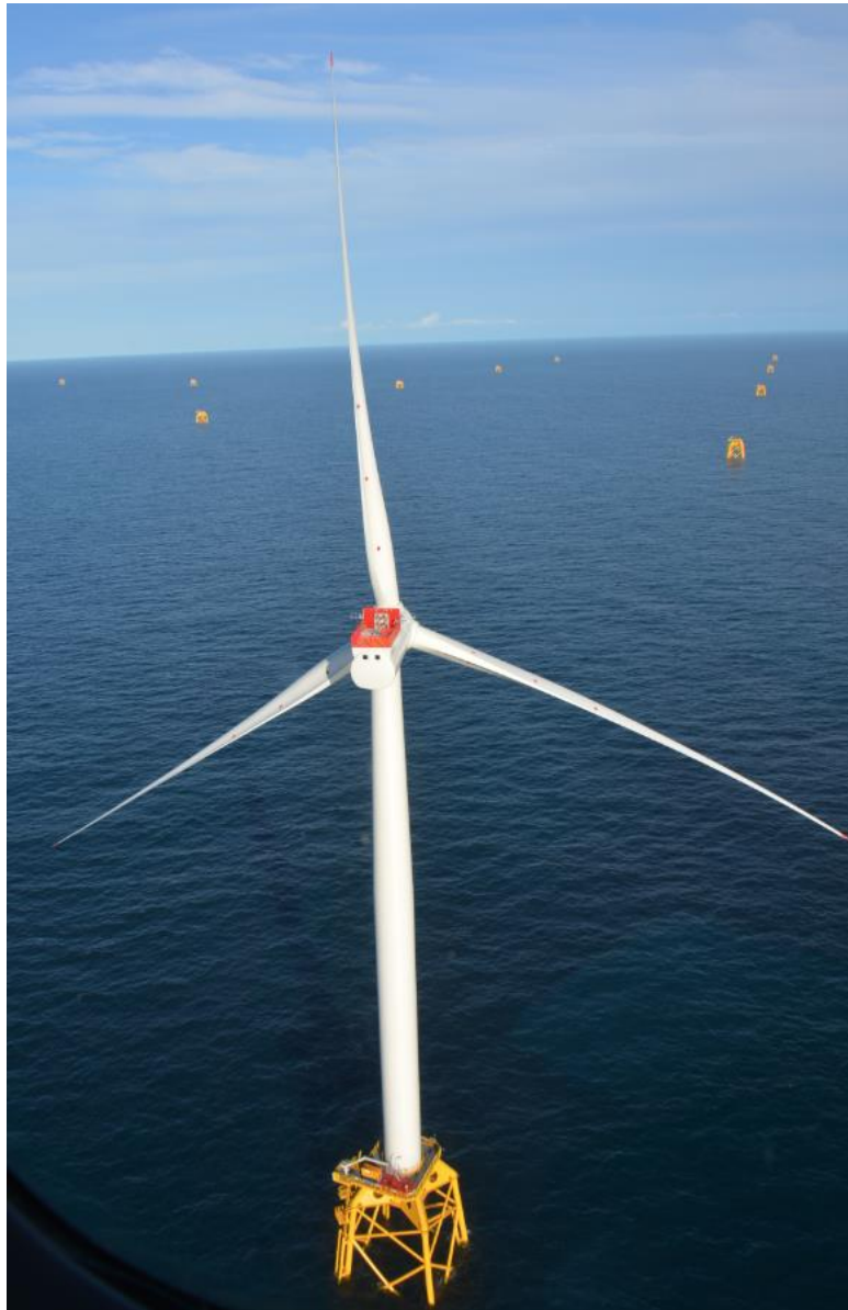
Fig. 5 Siemens SWT-7.0-154 WTG installed at Beatrice OWF
