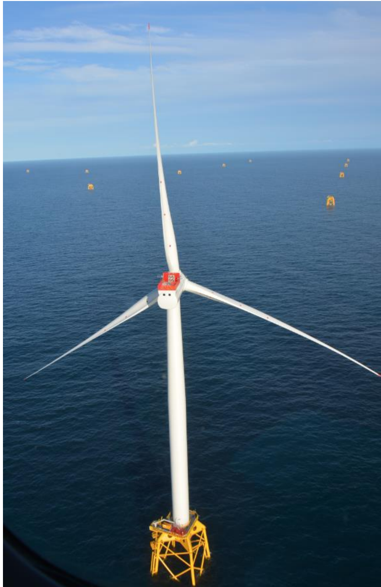
Fig. 5 Siemens SWT-7.0-154 WTG installed at Beatrice OWF
